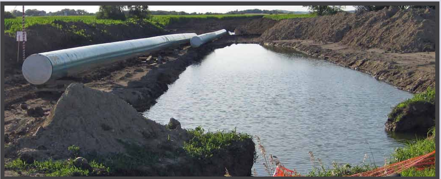
Keystone I pipeline under construction in South Dakota. Photo credit: Plains Justice.
